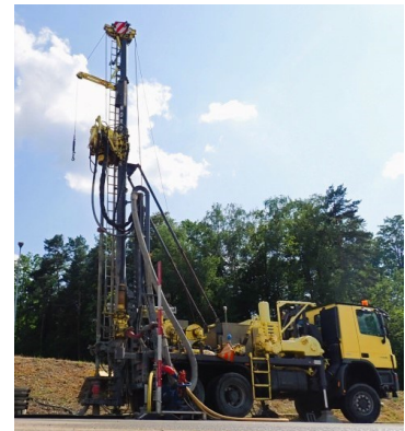
In the reporting year three exploratory drillings were conducted to explore the subterranean channel.
