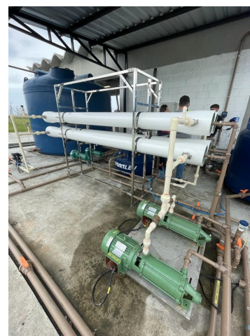
The reverse osmosis plant in Florianópolis
